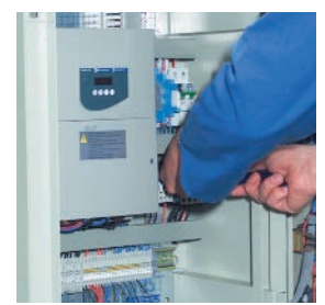
CONTROL PANEL WITH FREQUENCY IN INVERTER
